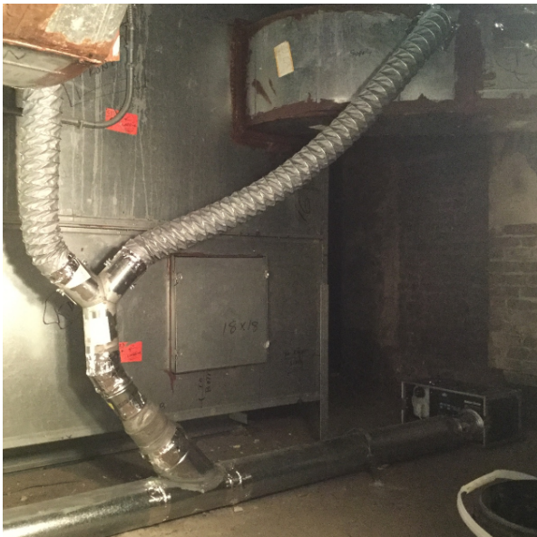
Figure 6 – Cowl Induction configuration could not achieve required static for induced flow in low velocity ductwork.
