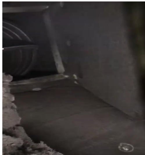
Figure 7 – GP microdroplets can be seen faintly in supply ductwork just downstream of GP injection point.
